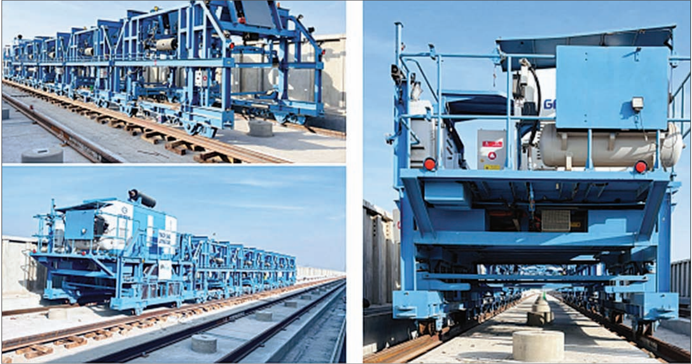
Track Slab Laying Car
