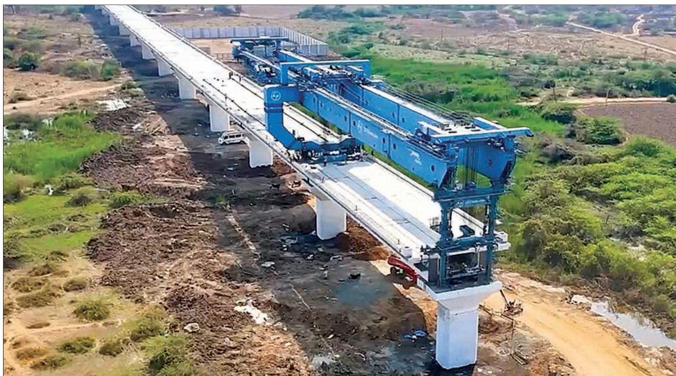
Girder Launching in progress using Full Span Launching Gantry, Surat District, Gujarat
