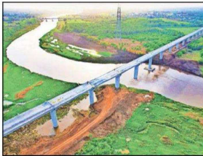
Aerial view of a bridge constructed by NHSRCL for Mumbai-Ahmedabad High Speed Rail Corridor, on Sunday. (ANI)
