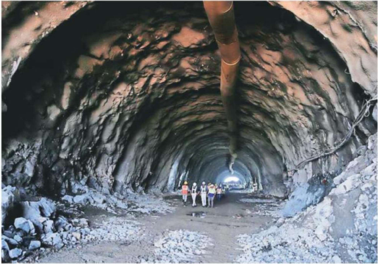
Breakthrough achieved in the first mountain tunnel of Mumbai-Ahmedabad High Speed Rail Corridor project, at Valsad in south Gujarat on Thursday. Photo courtesy: NHSRCL
