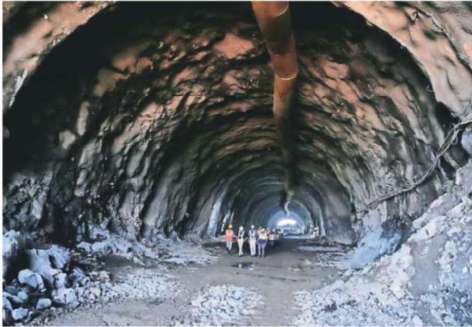
The breakthrough of the first mountain tunnel of the Mumbai-Ahmedabad High Speed Rail Corridor at Valsad in South Gujarat on Thursday. NHSRCL
