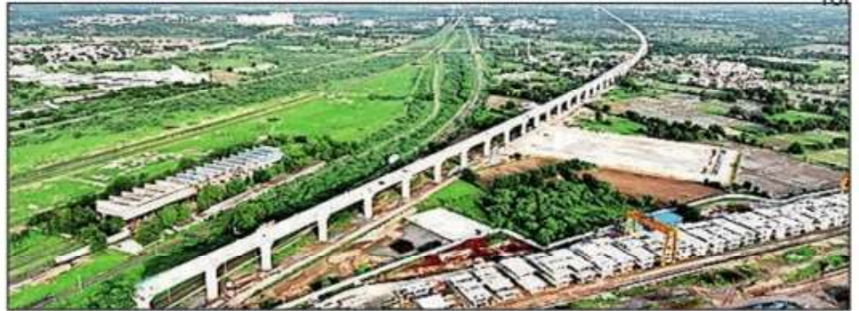
Construction work of Mumbai-Ahmedabad High Speed Rail viaduct in progress in Ahmedabad district
